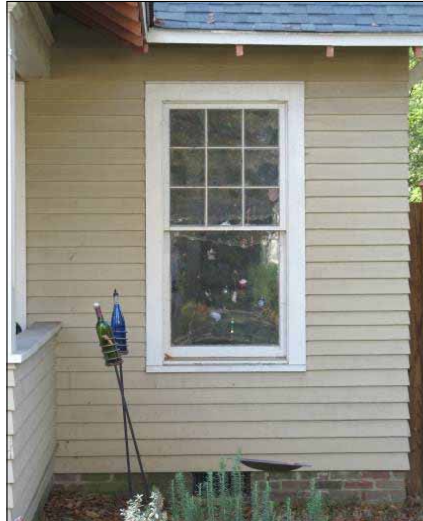
115 North Leflore Avenue uses beveled wood siding which is typical of the Craftsman style of architecture.
