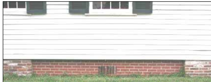
This homeowner at least recessed the new brick crawl space enclosure and included an air vent pattern in the bricks. This treatment would look more appropriate if the new brick were painted black and faced with lattice.
