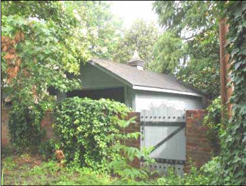
Historic outbuildings such as this historic garage (behind the wall) at 111 South Leflore Avenue should be preserved.
