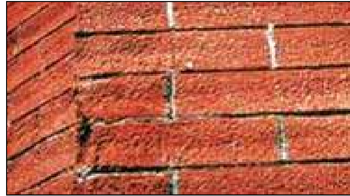
This National Park Service photograph well illustrates the negative effects of sandblasting, which should never be used to clean brick buildings. Sandblasting will not only erode mortar but will also remove the glazed outer surface of brick and hasten deterioration.
