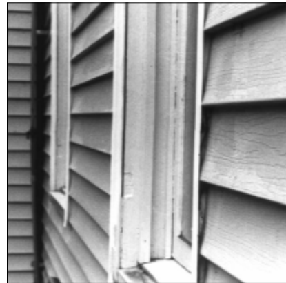
These photographs illustrate how vinyl siding negatively alters the exterior appearance of a historic building. The vinyl siding is nearly flush with the trim around the windows, and J-channels have been installed around the windows to prevent water infiltration behind the siding.
