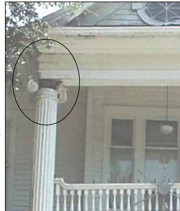
Failure to clean and maintain gutters is the primary cause of porch deterioration such as the damage caused to the column capital.
