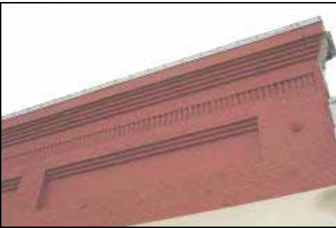
The brickwork of the parapets on several commercial buildings in downtown Cleveland feature decorative brick pattering and projecting bricks to give interest to the façade.
