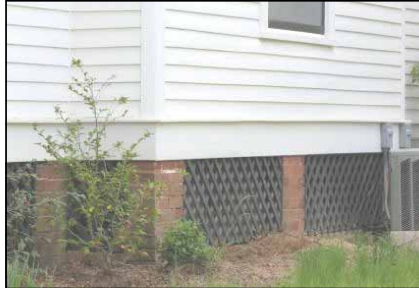
The lattice panels between the brick piers on this historic house appropriately enclose the crawl space area.
