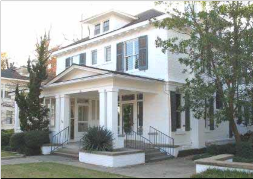
The house at 111 North Victoria Avenue has original louvered wood shutters that are operable and properly hang on shutter hooks.
