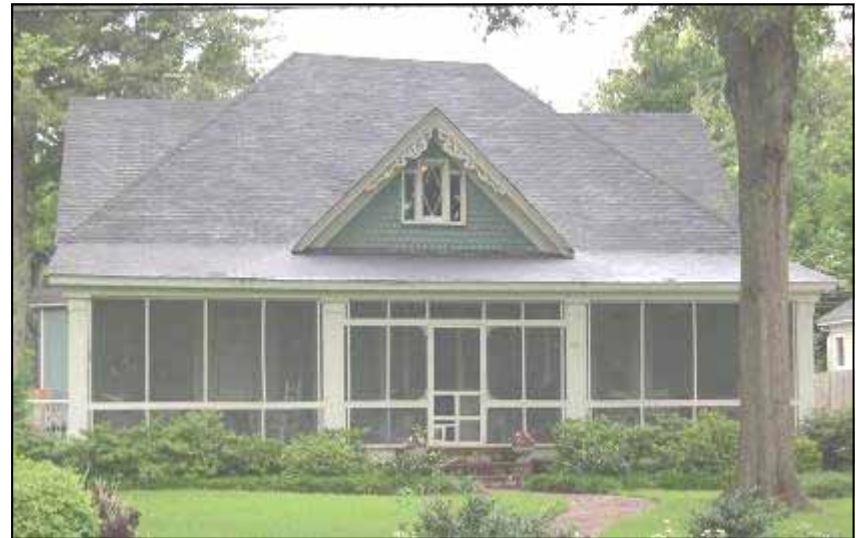
The original columns at 210 South Bolivar Avenue were most likely turned and later replaced with box columns.
