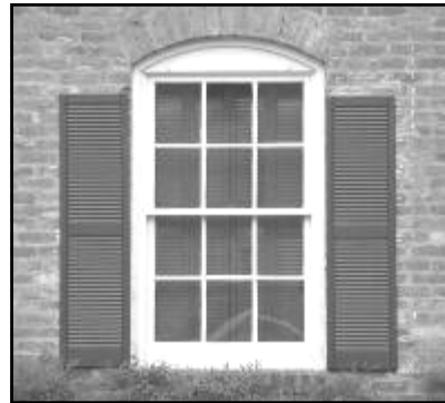
Shutters on this arched window are too short, too narrow, and wrongly hung outside the window frame. Shutters for this window should also form an arch when closed.
