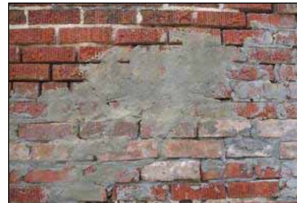
The owner of this brick building tried to stop the mortar erosion and water infiltration by smearing concrete over the deteriorated areas. This makes it very difficult to properly repair the problems in the future and has caused more damage to the brick surface
