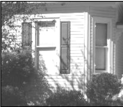
The vinyl shutters flanking this window are too narrow and incorrectly hung outside the window frame. Paneled shutters are also inappropriate for Queen Anne style houses.
