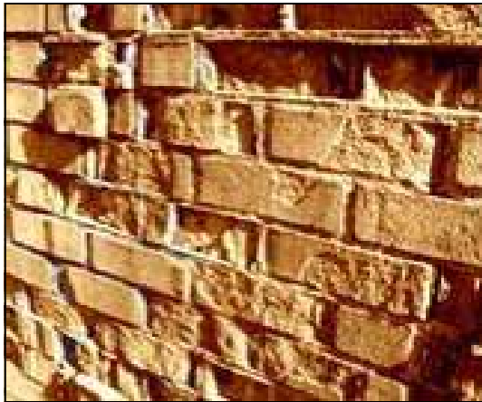
This photograph supplied by Chagrin Falls Preservation in Ohio illustrates the spalling that can occur only five years after using portland cement mortar in repointing.
